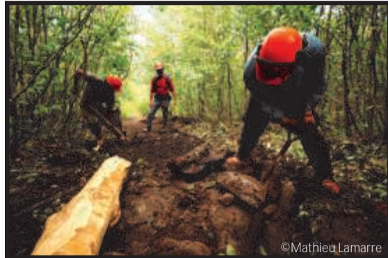
The construction of a new trail section; Mahican Diamond, Jean Lacasse and Matthew Cleary are at work.
